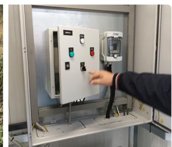
Solar fixture control panel (c) City of Zagreb
