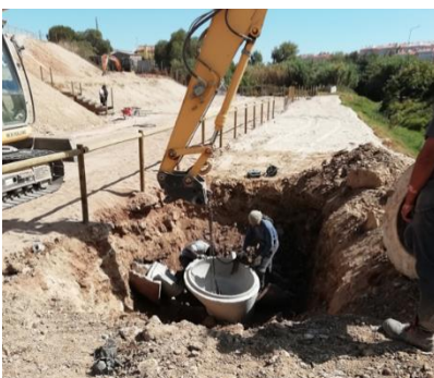
Ensuring access to rainwater pipes. Source: Coscais Ambiente
